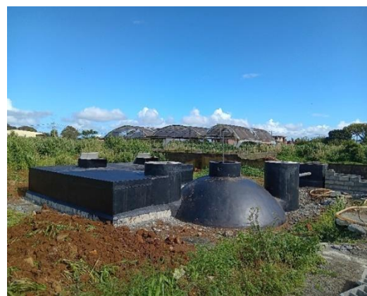
Figure 39: Wasaza fixed dome biodigester at Curepipe LRS
