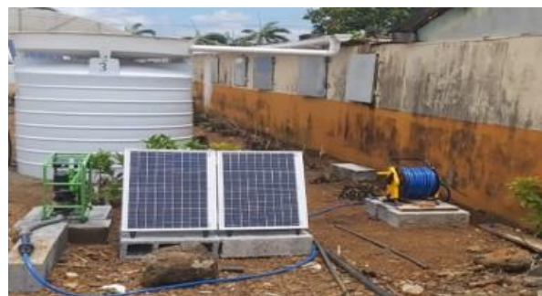
Figure 26: The Rainwater Collecting Tank with the SF-2 Futurepump Solar Power-Driven Pump
